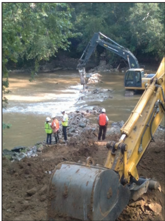
Bulldozers and jackhammers were used in the removal of the dam at Lassiter Mill on the Uwharrie River.
