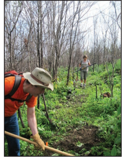
Join us as we restore lost sections of the historic Uwharrie Recreational Trail!
